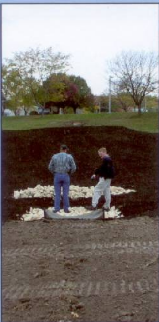
Application of compost to a storm water basin improves water holding capacity and infiltration.
